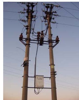
Pole mounted FTU
