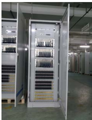
RTU for Substation
